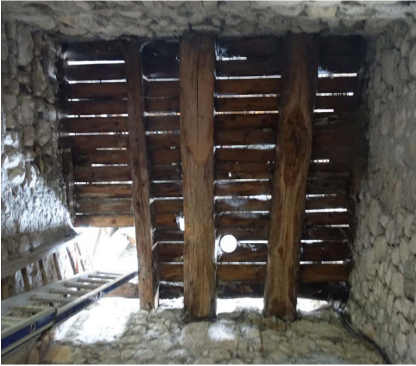
Plancher clocher - solives saines
